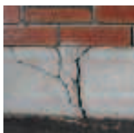
Cracks in foundation walls
