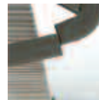
Leaky rain gutter
