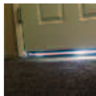
Gaps under doors
